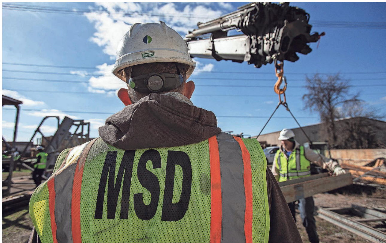
A MSD crewmember operated a remote-control crane while training on the installation of floodwall enclosures at the MSD central maintenance facility on Cane Run Road on Tuesday morning in February in Louisville. The training exercise replicates portions of MSD's flood-protection system, which includes 26.1 miles of floodwall.
